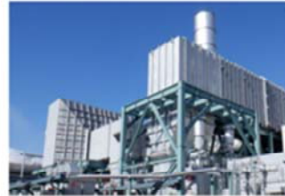
Mitsui Chemicals' high-efficiency gas turbine power generation system
