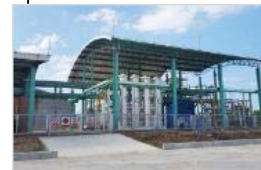
Biogas Upgrading System (Thailand)
