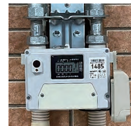
Smart meter with communication unit
