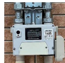
Smart meter with communication unit
