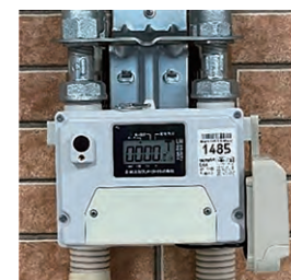
Smart meter with communication unit
