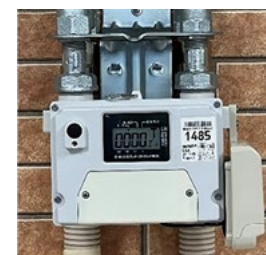
Smart meter with communication unit
