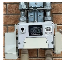
Smart meter with communication unit and repeater
