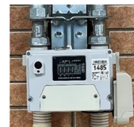
Smart meter with communication unit
