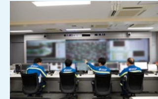
Supply control and irregularity monitoring
