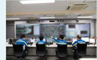
Central Control Room
