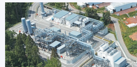
Sabatier methanation demonstration facility in Nagaoka Courtesy of INPEX
