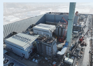
Himeji Natural Gas Power Plant
