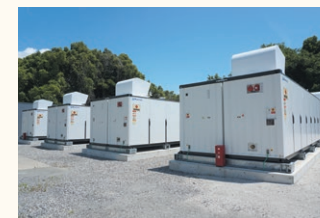
Senri Power Storage Plant
