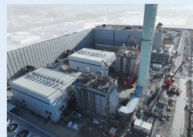
Himeji Natural Gas Power Plant
