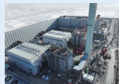
Himeji Natural Gas Power Plant
