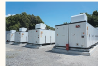
Senri Power Storage Plant
