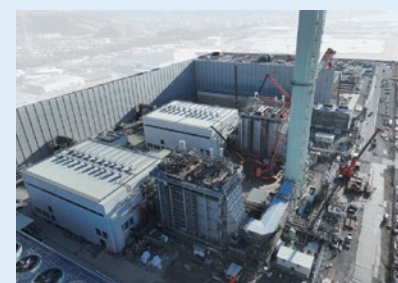
Himeji Natural Gas Power Plant
