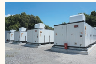
Senri Power Storage Plant
