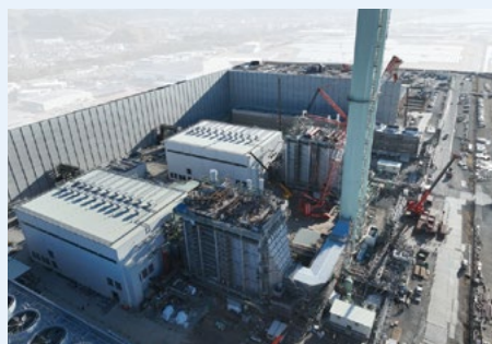
Himeji Natural Gas Power Plant
