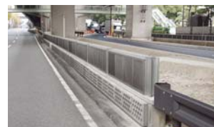
Activated carbon filter (ACF) installed beside major thoroughfare
