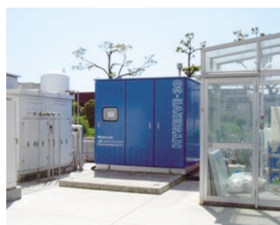
HYSERVE 30* set up in the hydrogen filling station in the Osaka Gas field lab.
