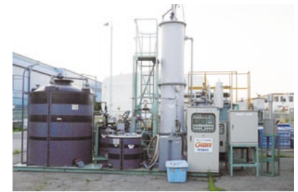
Pilot plant for the noxious effluents treatment and the biogas generation
