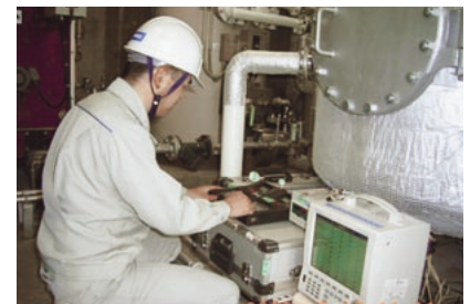
Energy saving diagnostics
