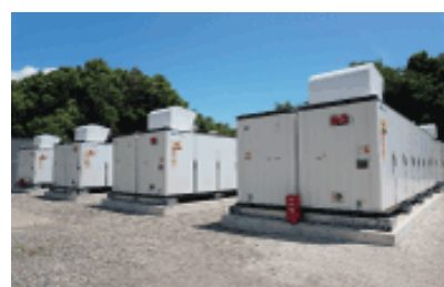
Senri Grid Storage (Osaka Prefecture)
