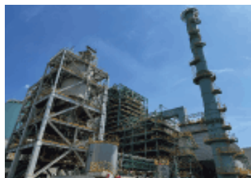
Wakayama Gobo Biomass Power Plant (Wakayama Prefecture)
