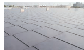
Torishima Solar Power Plant
