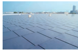
Torishima Solar Power Plant (Osaka Prefecture)
